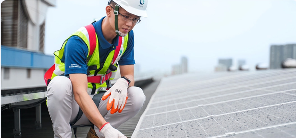
SP is installing rooftop solar PV systems at six of AA REIT's properties
